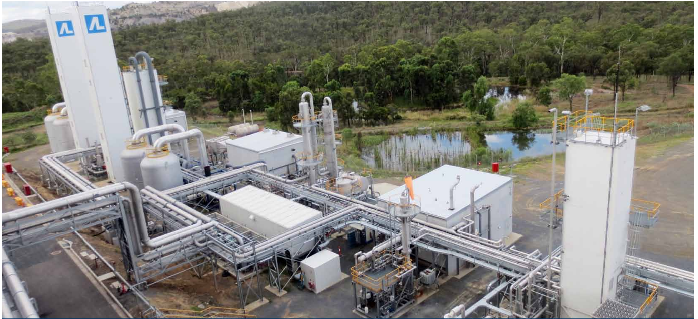
The completed air separation unit and carbon dioxide processing unit on the Carbon Dioxide Capture Plant.
